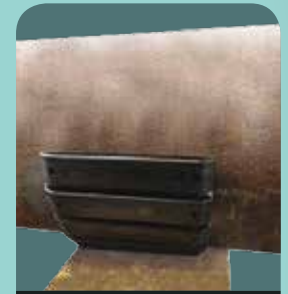
Pipe on support
